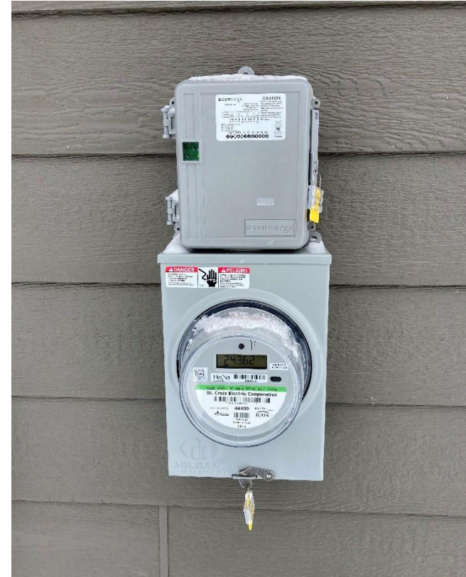
Example of off-peak installation – meter supplied by SCEC
